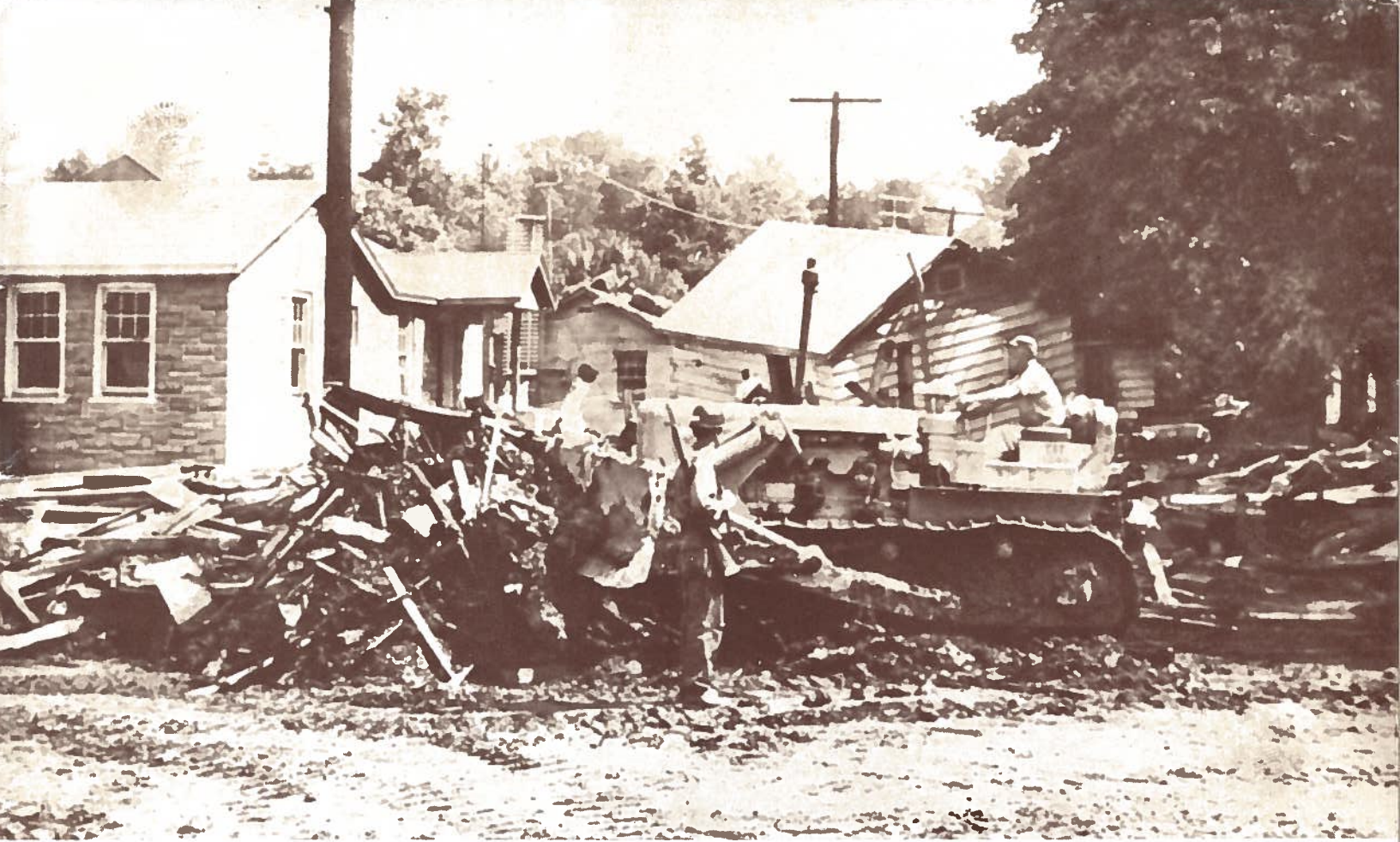
WHILE AN ARMED NATIONAL GUARDSMAN looks on, a bulldozer clears away some of the flood debris in Stroudsburg as the community continues its mop-up operations in the wake of the flood. In background is a house carried off its foundations by the flood waters.
