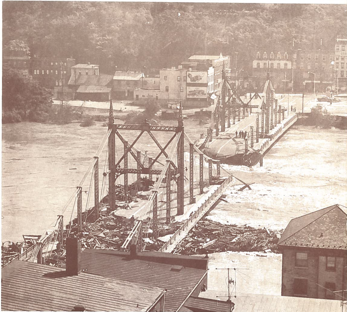
07-29-52 L 13 1/2 A LIFELINE IS CUT between Easton, Pa., and Phillipsburg, N. J., as the raging flood hammers a great gap from the Delaware River free bridge.
