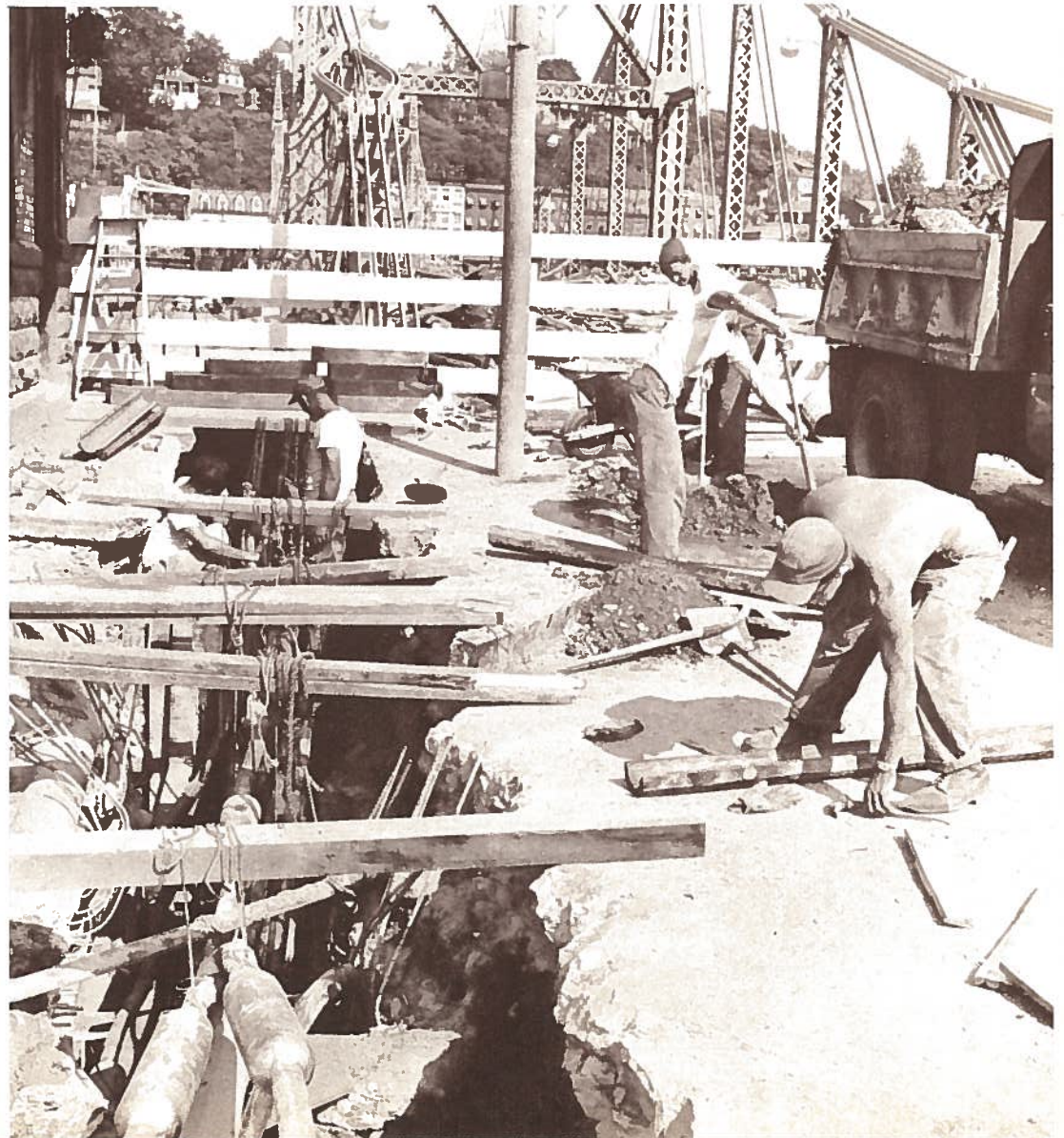
BELL EMPLOYEES CONNECT CABLES at Front and Northampton streets. In the background are barricades across the entrance to the washed-out Northampton street bridge.
