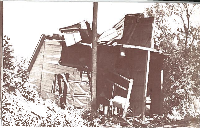
BOTTOMS UP AT CARPENTERSVILLE, N. J., as the Delaware River, tickled by Hurricane Diane, plays tricks with a summer cottage.
