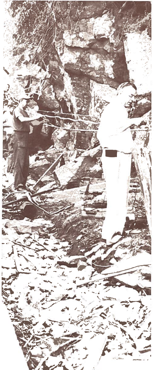
TELEPHONE LINES are restored on an emergency basis along Route 611 south of Easton.
