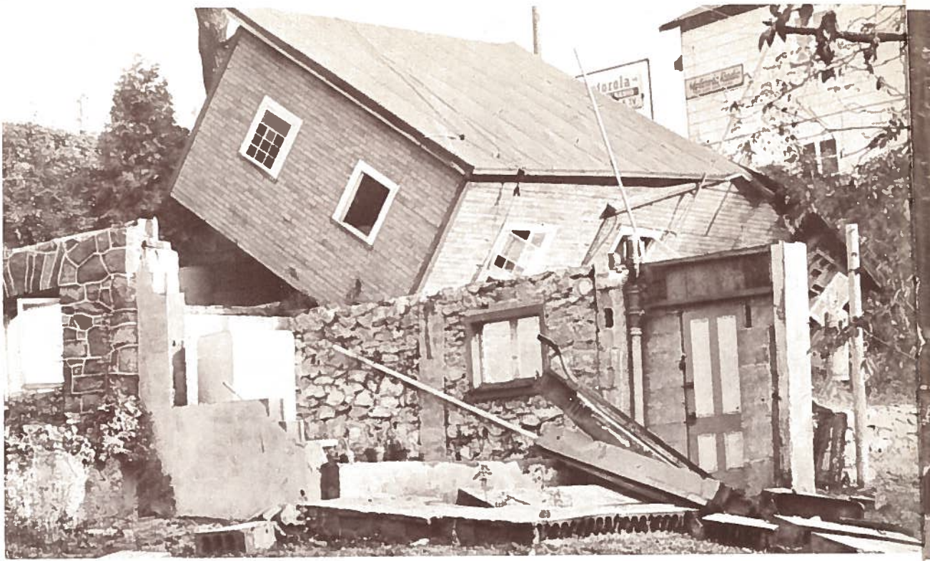
THE SECOND FLOOR AT the cottage of Mr. and Mrs. Joseph A. Amoroso, North Delaware drive, Easton, is shown here tilted at nearly a 45-degree angle.
