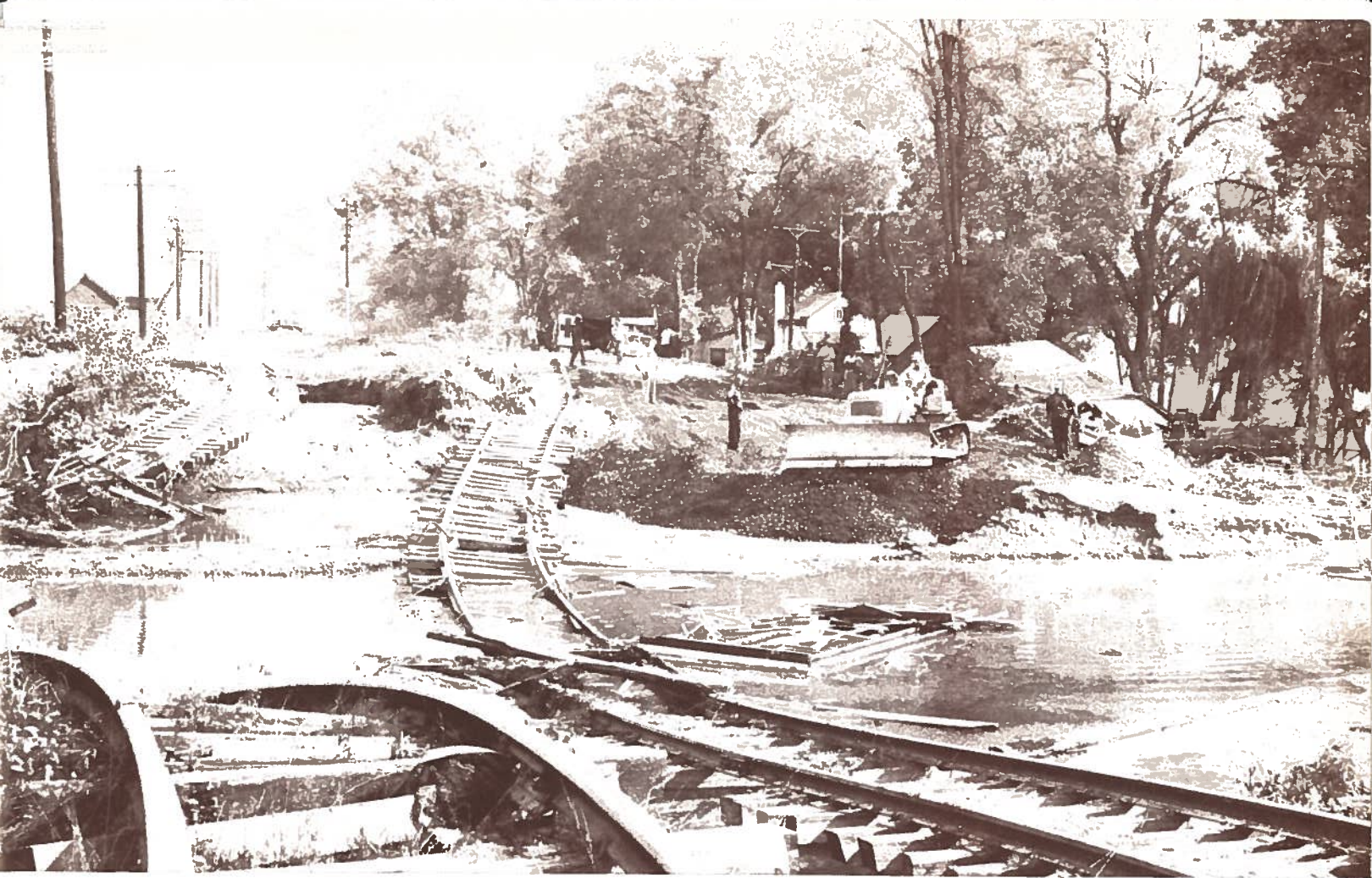
TWISTED STEEL RAILS OF THE PENNSYLVANIA railroad at Carpentersville, N. J., testify to the force of the Delaware River flood.
