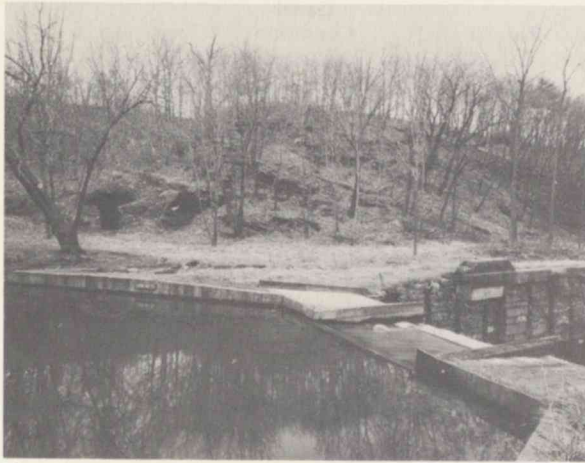
Near Weissport, Lock 10 is stabilized and maintained by the Lehigh River Restoration Association.
