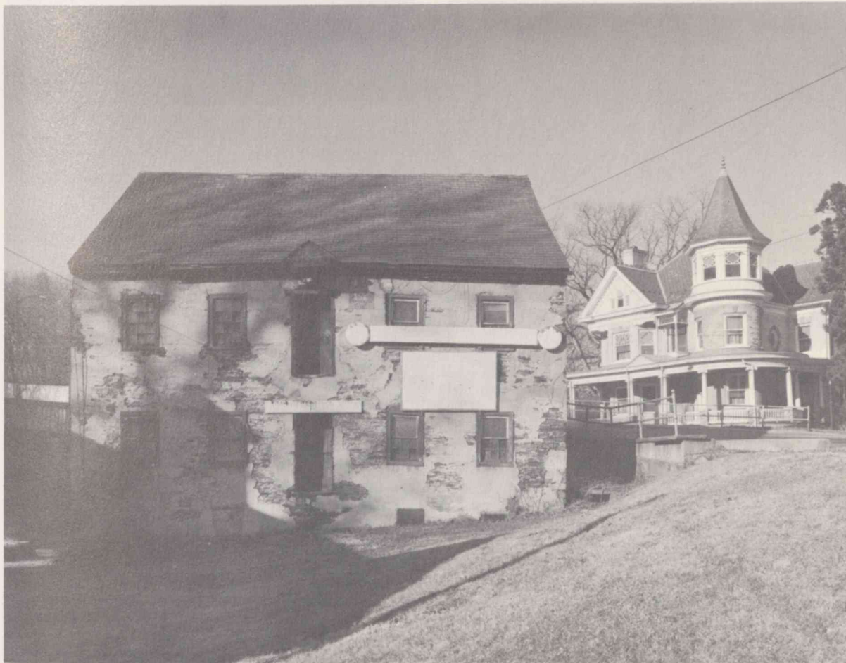
The Kern Roller Mill, built in 1859, used slate as its primary construction material. Slate structural details may be seen in buildings throughout the town.
